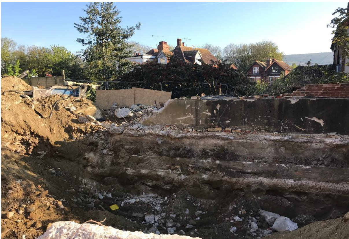
Plate 4: Showing construction cut of recently demolished building/ tank. The truncation clearly reaches depth of nearly 3 meters below existing ground level. Photograph kindly provided by demolition team.
